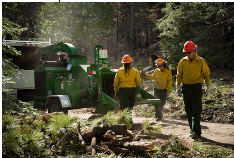
Tahoe Conservation Partnership Crews chip wood as part of a forest improvement project.
