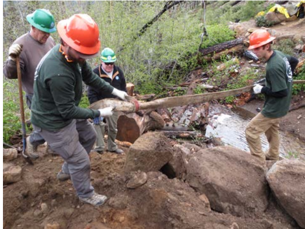
TRCD Crew during Heavenly Creek Bridge Construction at Van Sickle Bi-State Park
